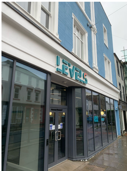
Photograph 4 Oblique view showing tray depth and the apparent interruption of the fascia moulding.
